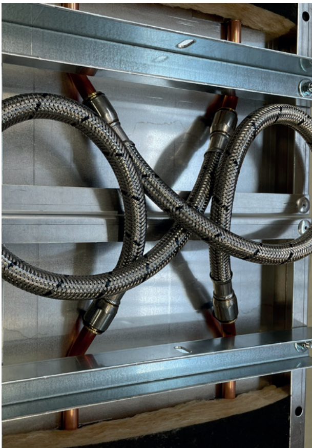
Figure 13. A pair of interconnecting hoses between panels
