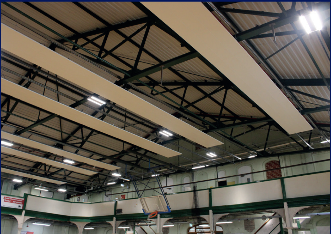
iTwelve Industrial Radiant Panels installed at St Mary's Community and Leisure Centre, Southampton.
